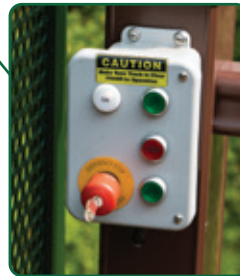
Control box at top and bottom of track with security lock.
