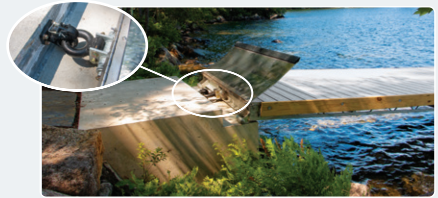
Concrete anchor pad with aluminum tread plate and pintle hitch.
