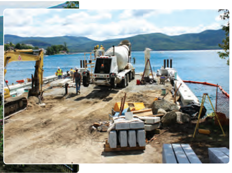
Above: Complete waterfront restoration including pier replacement and new commercial pile docks.
