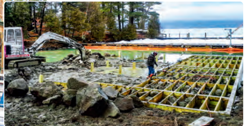
Below: New crib dock as a foundation for the boathouse shown left.
