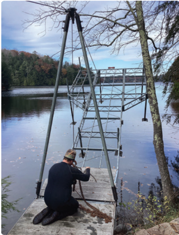
Above: One of our employees raising an articulating dock for winter storage.
