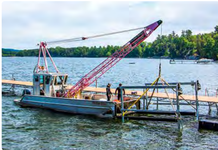
Ultimate lift being installed by one of our crews using our portable workboat "Miss Doc".
