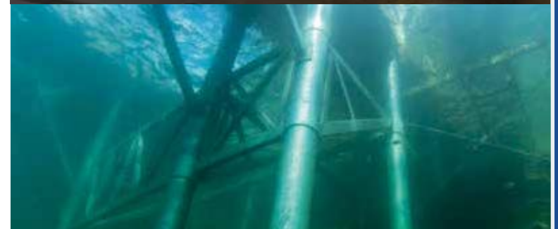
Underwater view of the dock installed in area with a steep drop-off and heavy exposure. Includes underwater bracing and 4,800 lb. anchor blocks.
