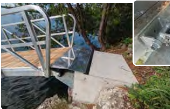
Concrete anchor abutment with aluminum tread plate and pintle hitch.
