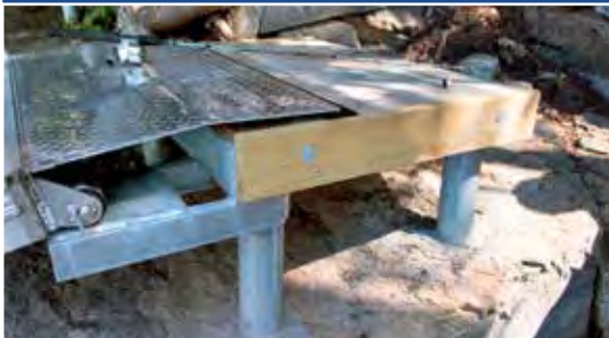
Our pile platform as a shore anchor for gangway and floating dock.
