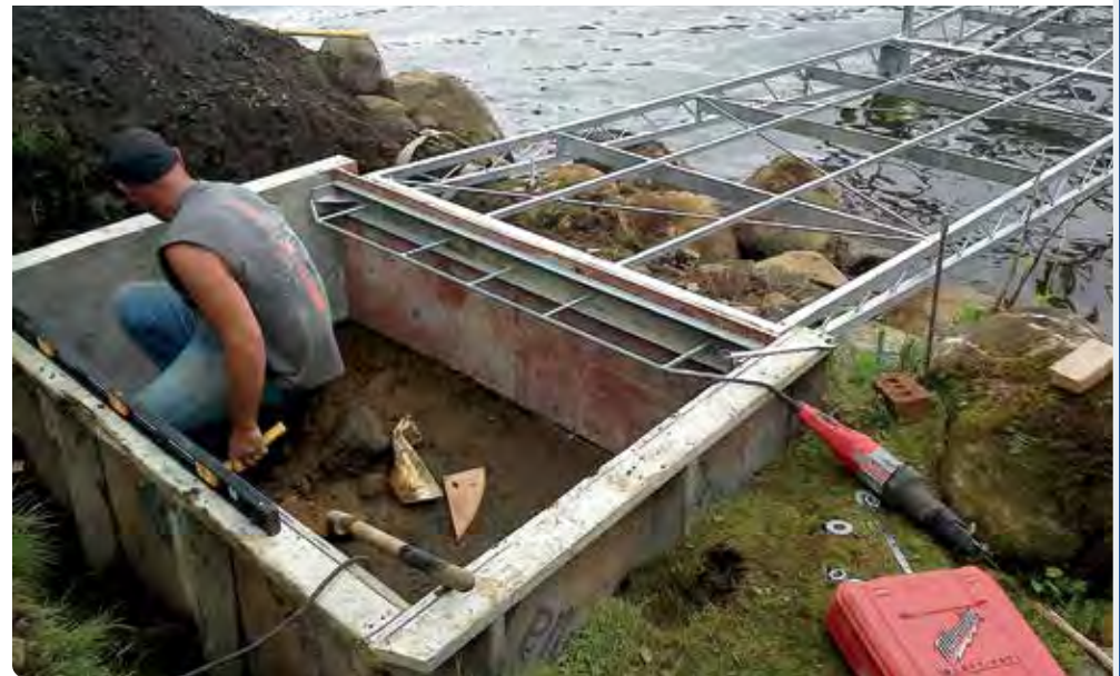
Above Top: Articulating dock with a concrete abutment as a shore anchor. Above: Forms being assembled for the concrete abutment.
