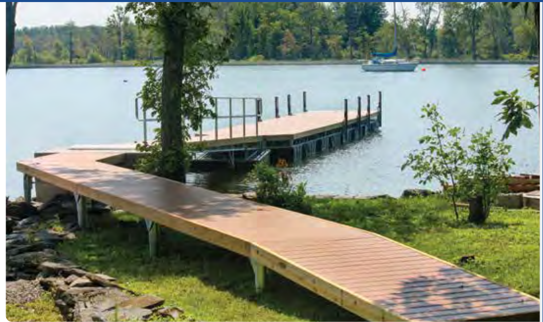
Pile dock sections used as an elevated walkway to gain access to the floating dock during high water events.
