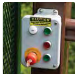
Control boxes at the top and bottom with security locks.
