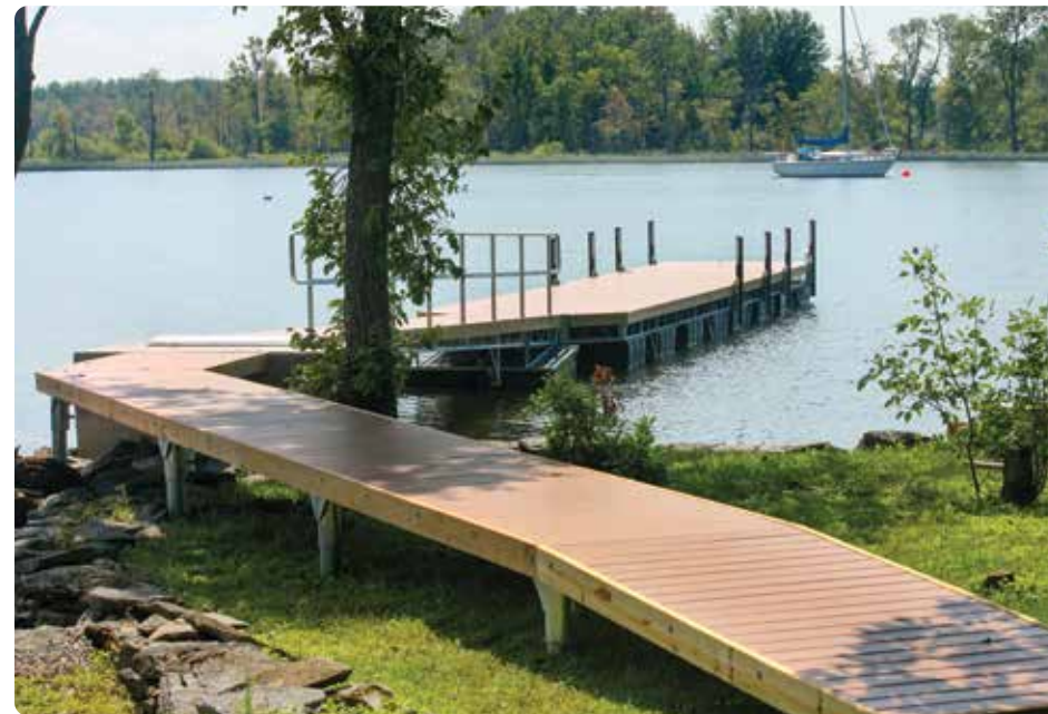
Pile dock sections used as walkway to transition over a wetland area to main floating truss dock.
