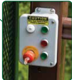
Control box at top and bottom of track with security lock.
