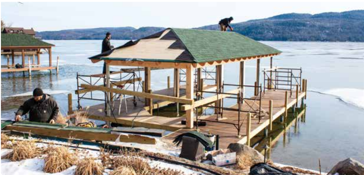
Our U-shaped pile dock serves as the foundation for the above open-sided boathouse. Above: Boathouse in final stages. Above Top: Boathouse completed.
