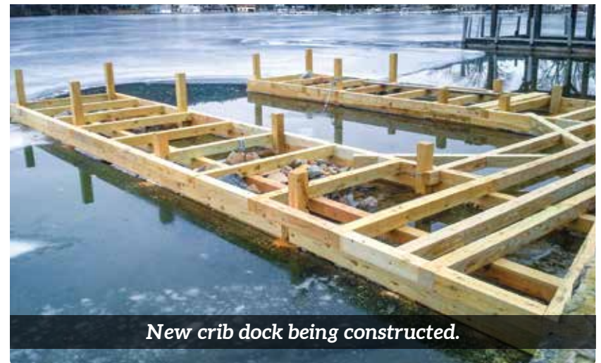
Crib dock foundation completed with boathouse uprights in place for sundeck construction.
