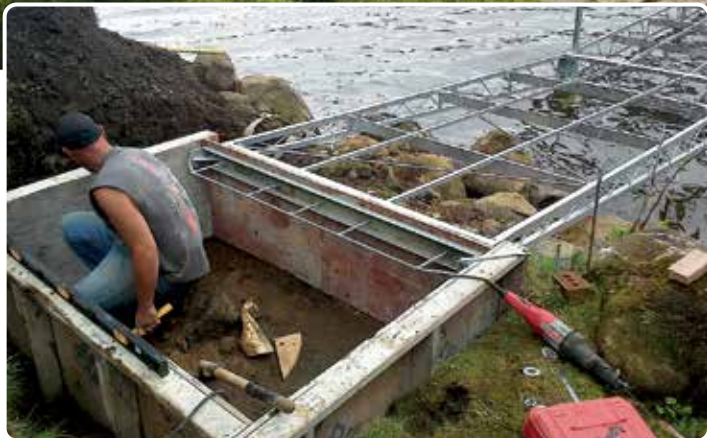
Above Bottom: A concrete pad is being formed to serve as the shore hitch for the above articulating dock.
