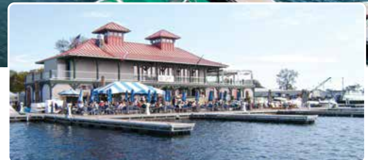
Commercial steel truss floating system installed at the Burlington Boathouse, Burlington, VT
