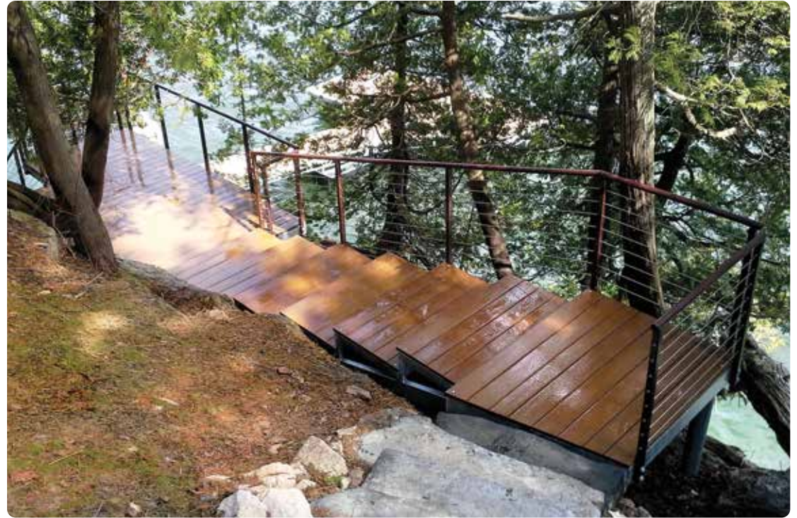
Stainless-steel cable rail provides safety and an open aesthetic appearance.
