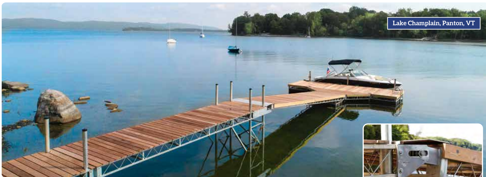
Above: Our mega-duty leg dock used as a transition to a custom steel truss floating dock for a site that has high spring water levels. Inset: Close up of the connection from the leg dock to the floating dock.
