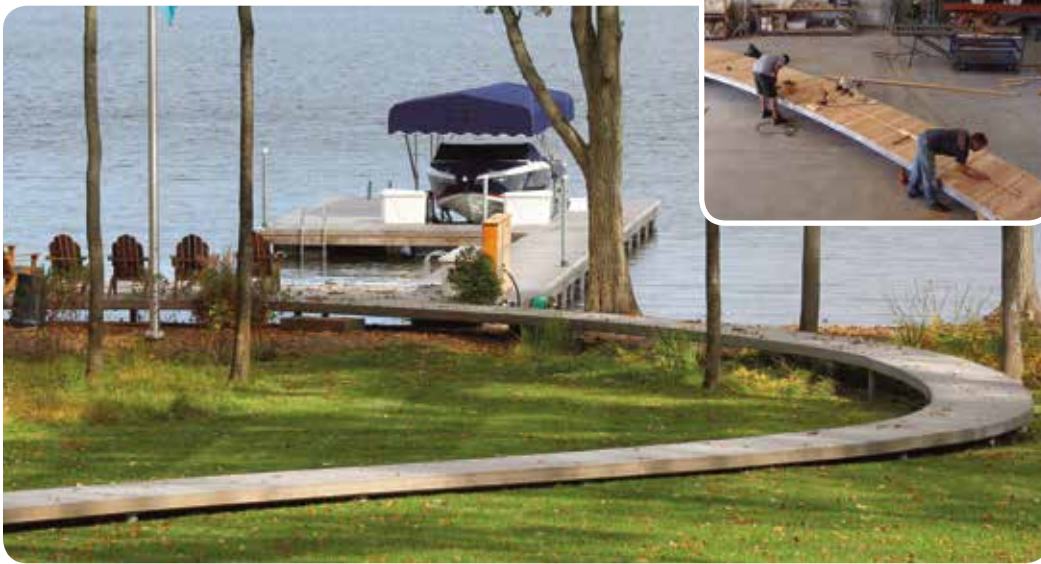
Above: Curved walkway using our galvanized steel permanent pile platform. Inset: During fabrication in our workshop.
