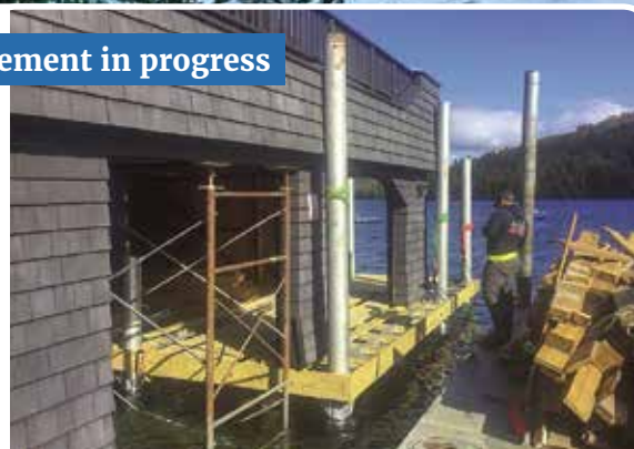
Left: Lifting and supporting the boathouse structure prior to foundation removal and replacement. Right: Installation of new pile dock foundation.
