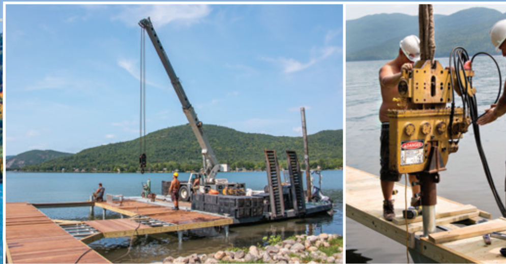
Piles are driven into the lakebed with our workboat and pile driver
