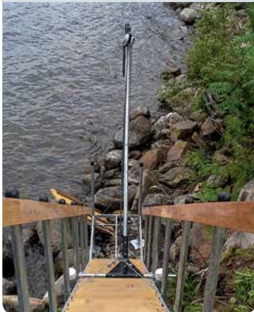
T-pole lift system in place ready to raise lower stair section for winter storage.
