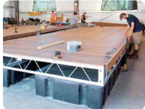
Final decking being installed on a commercial dock section at our production facility.
