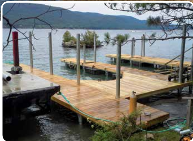
Pile dock foundation in place with extended upright supports for boathouse. (Above: Boathouse by others completed.)
