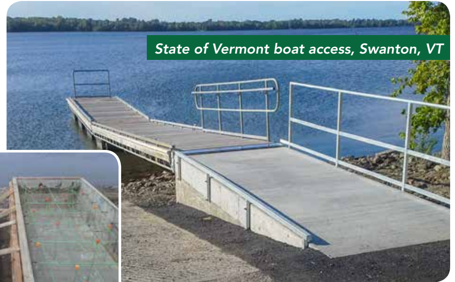
ADA concrete access ramp with handrail & our galvanized steel truss floating dock with ADA curbing.
