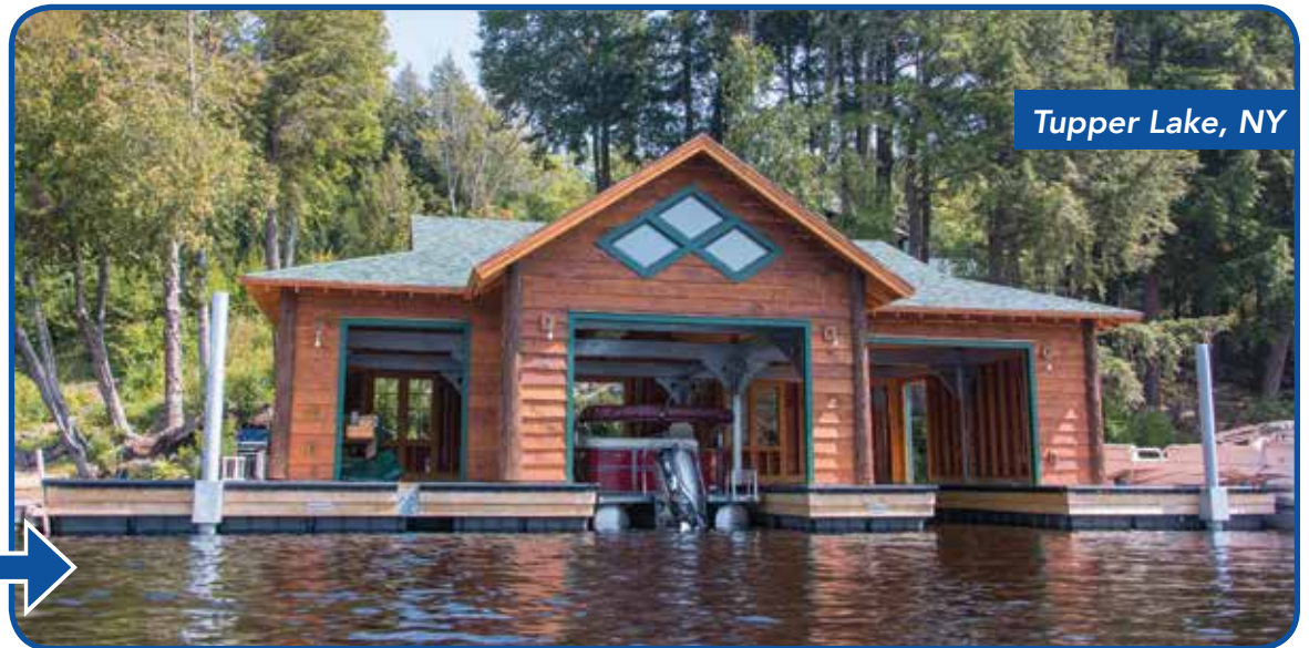
Bottom Left: Floating foundation and boathouse support structure being erected on site. Above: Completed boathouse (wooden boathouse structure by others).
