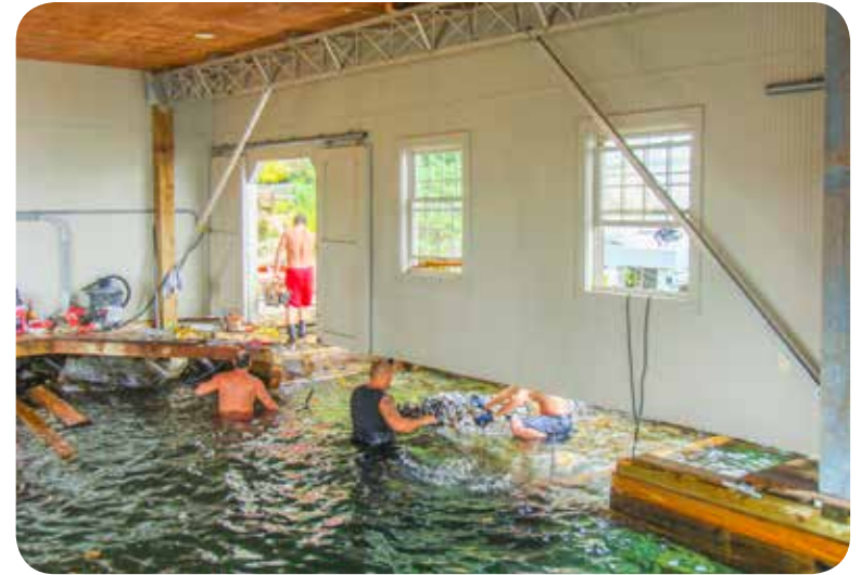
Above: Crib dock foundation being removed in preparation for a new pile dock foundation.
