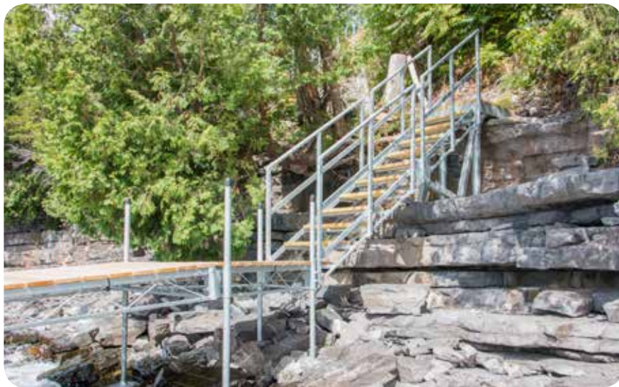
Stairs with lower platform that connects directly to our steel truss leg dock.
