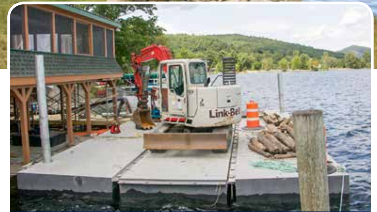
Our sectional barge and excavator can reach sites with little or no shoreline.
