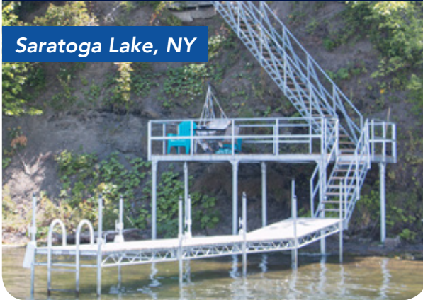
Shoreside platform used as a transition for the steel stair system and waterfront deck area for a site with no beach.
